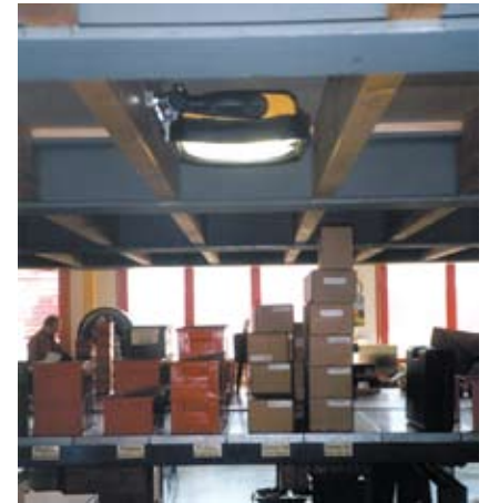
Optimum workstation lighting using PRIMA light, dazzle-free ceiling light with significant light output with low heat formation.
